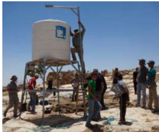
Figure 2: COMET-ME water holding tank
