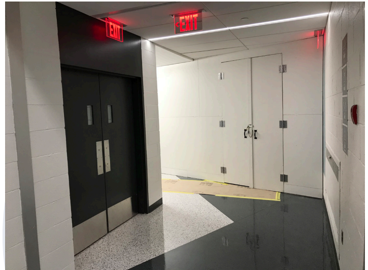
The temporary construction barrier installed on the second floor of the Frable Building.
