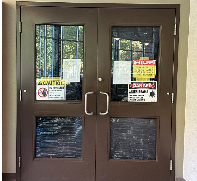
The office suite in the basement of the Student Community Center (SCC) is being remodeled to open in time for Spring, 2023 (Photo courtesy: Carlin Whalen)
