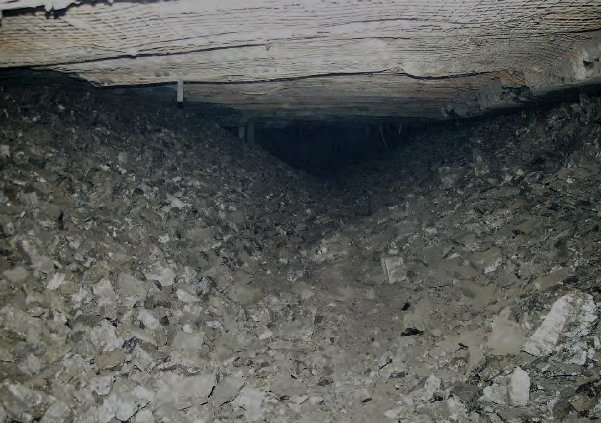
South Barrier 4entry Looking inby CC119 ½ in #4 entry, 8/9/07 –Bump Damage
