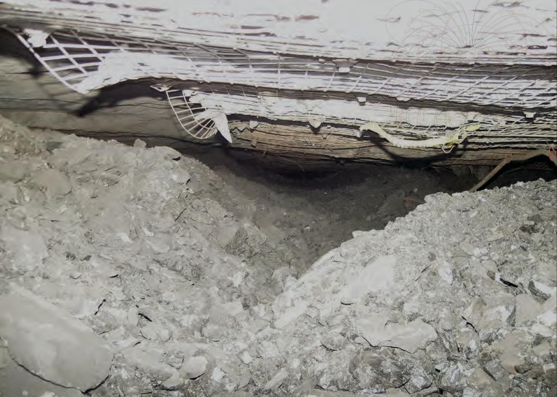
South Barrier 4entry Looking inby CC120 in #3 entry, 8/9/07 – Bump Damage
