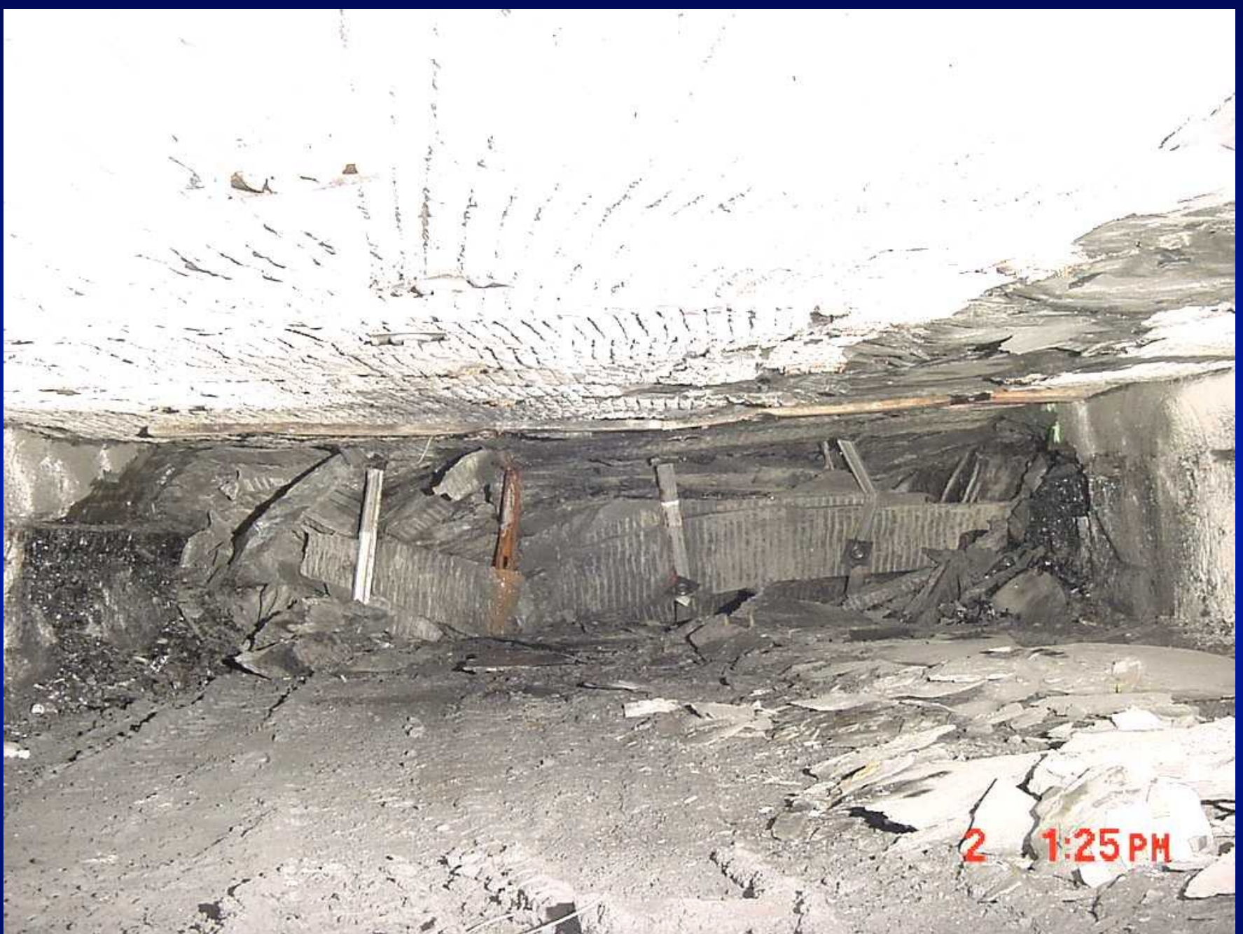
ROOF FALL INVESTIGATION
