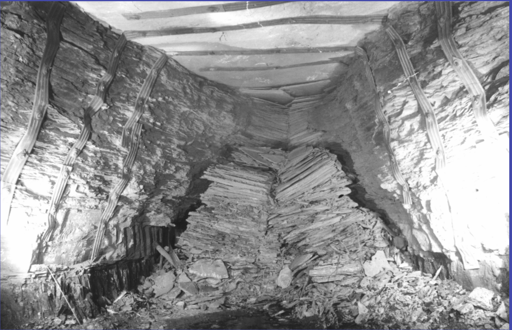
Roof Falls Above Anchorage
